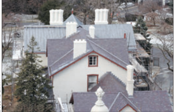
Wagner Roofing is installing a new Vermont slate roof and a standing-seam, lead-coated copper roof on the cottage.
