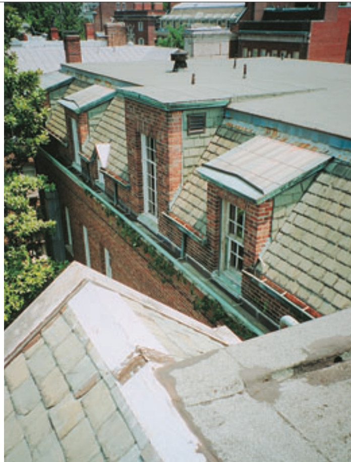
The L-shaped residence is surrounded on all sides by a slate-covered mansard roof, with dormers punched through around the entire perimeter.
